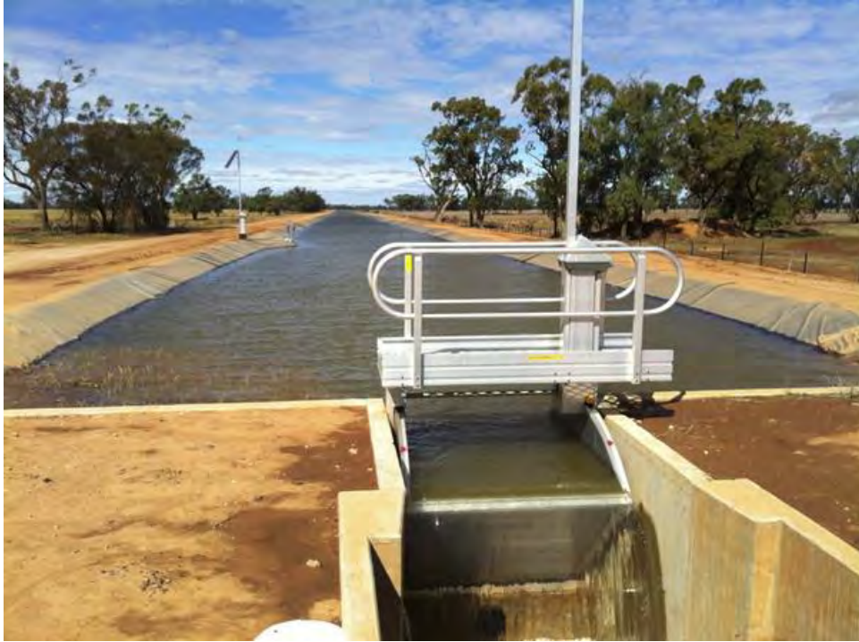
Photo 1. Lined channel section with Rubicon control gates.
